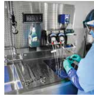
Sink stations optimized for each user, and each IFU requirement
